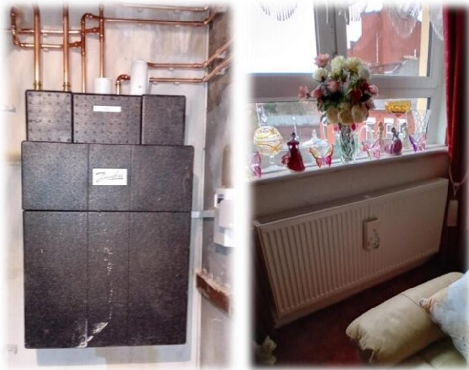
Pictures Above: New Heat Interface Unit & Radiators at Radnor House
