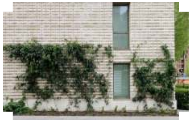
Vertical greening integrated up the walls of end terraces | Elephant Park, London
