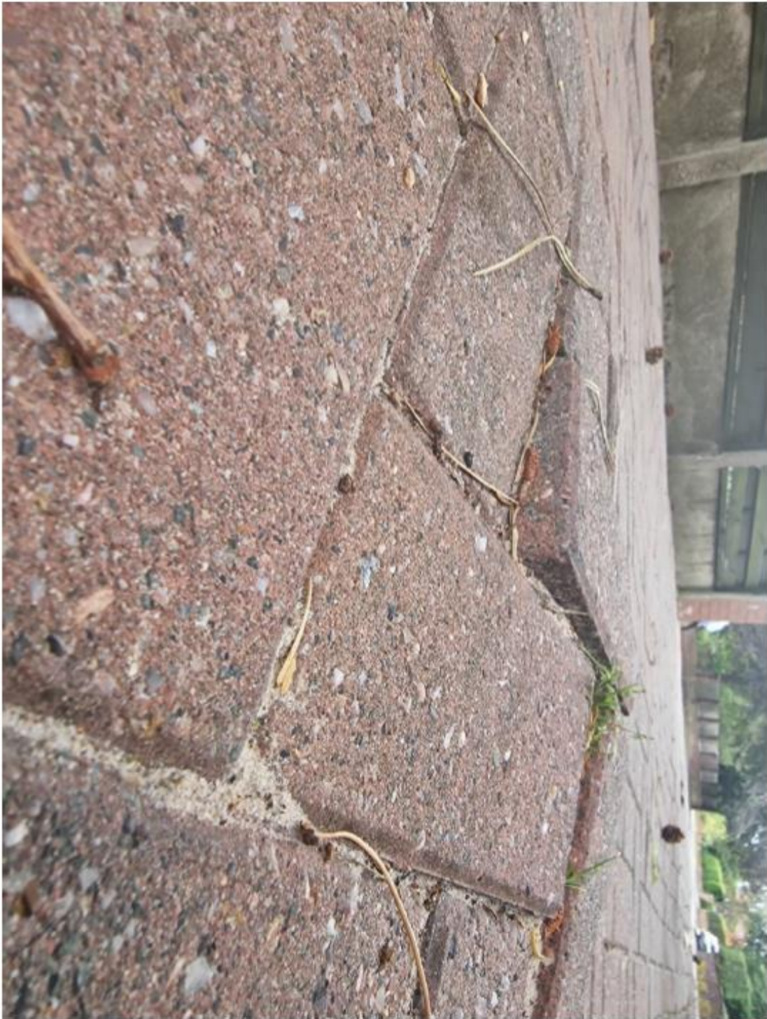
4: : Photograph illustrating root damage to driveway – closeup 1
