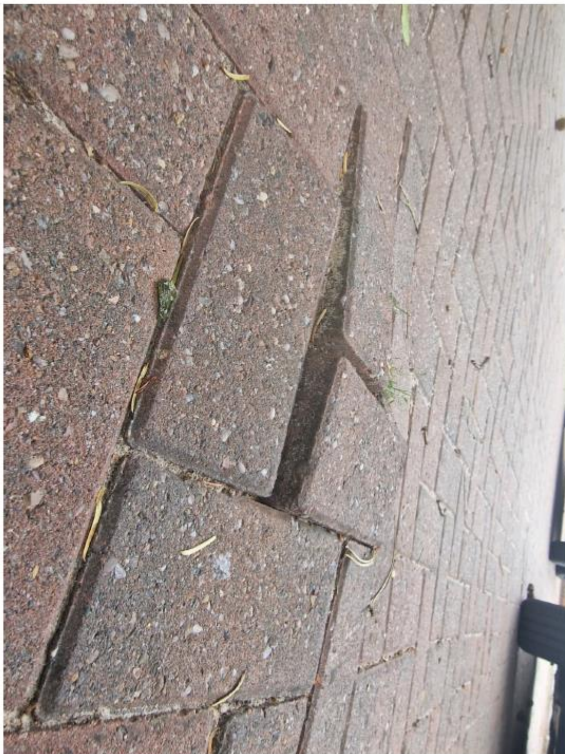
5: Photograph illustrating root damage to driveway – closeup 2
