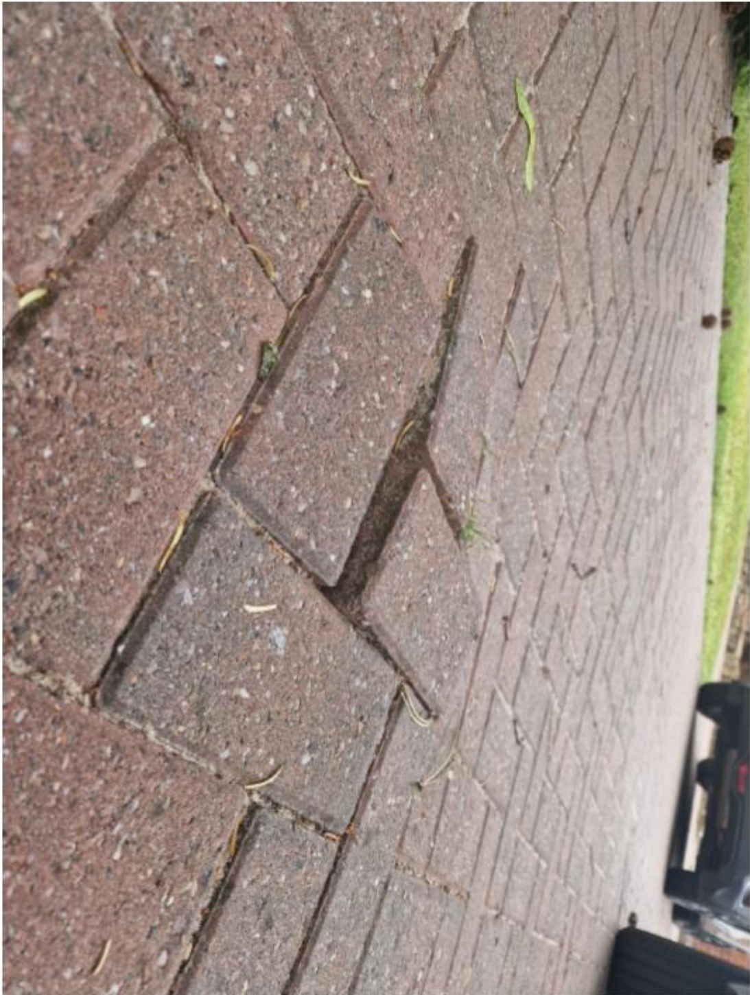
6: Photograph illustrating root damage to driveway – closeup 2
