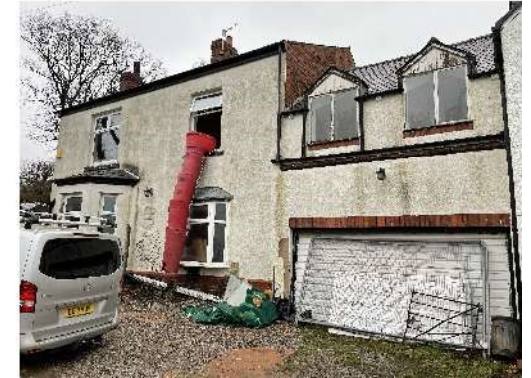
EXISTING FRONT SHOWING POORLY DESIGNED HIDEOUS DORMERS AND POOR QUALITY BUILD
