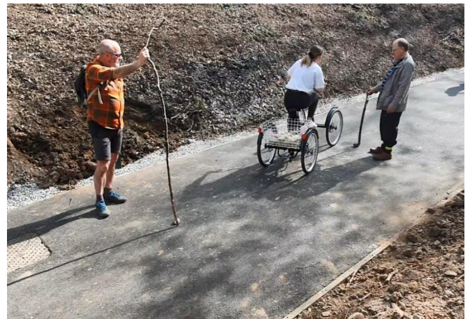
3.5m spacing of chicanes on a 3m path on a steep uphill as per Sustrans guidance. Picture shows 4 wheel pedal cycle
